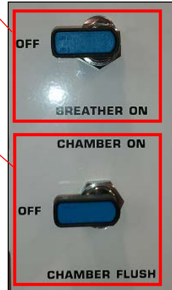
Figure 9: Oxygen Flow Control Panel
